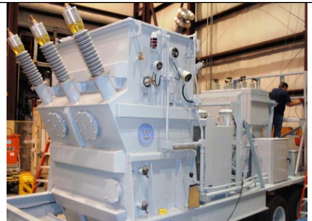
12 MVA 69 - 34.5Y x 13.8Y x 12.47Y Westinghouse
