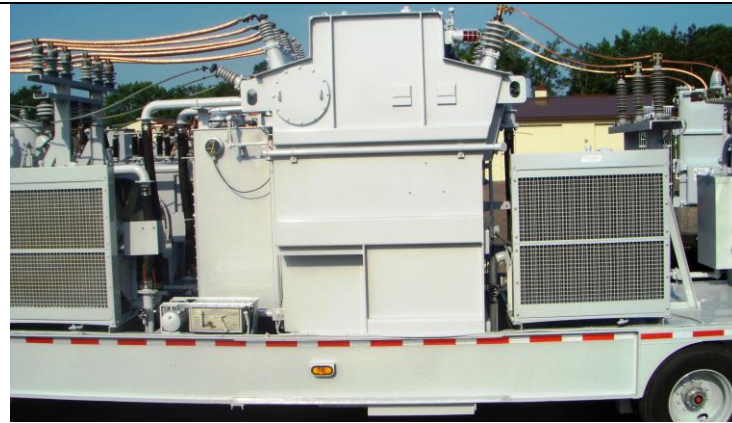
24 MVA 34.4 - 13.2Y LTC Westinghouse
