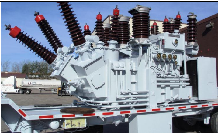
20 MVA 110Y x 69Y - 69Y x 34.5Y - 12.5 Westinghouse
