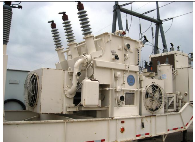
20 MVA 67 – 13.8Y Westinghouse
