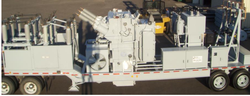
14 MVA 69 - 13.2Y Westinghouse with new Reinhausen LTC
