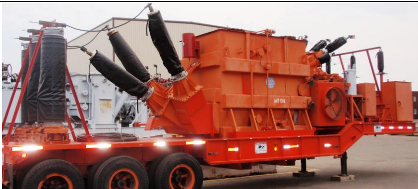
44.5 MVA 161Y x 115Y - 69Y Westinghouse Auto
