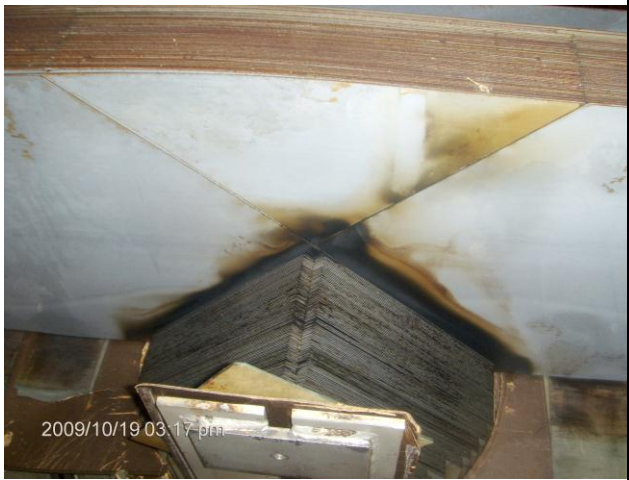
Overheated Sheets of Center Leg Top Yolk
