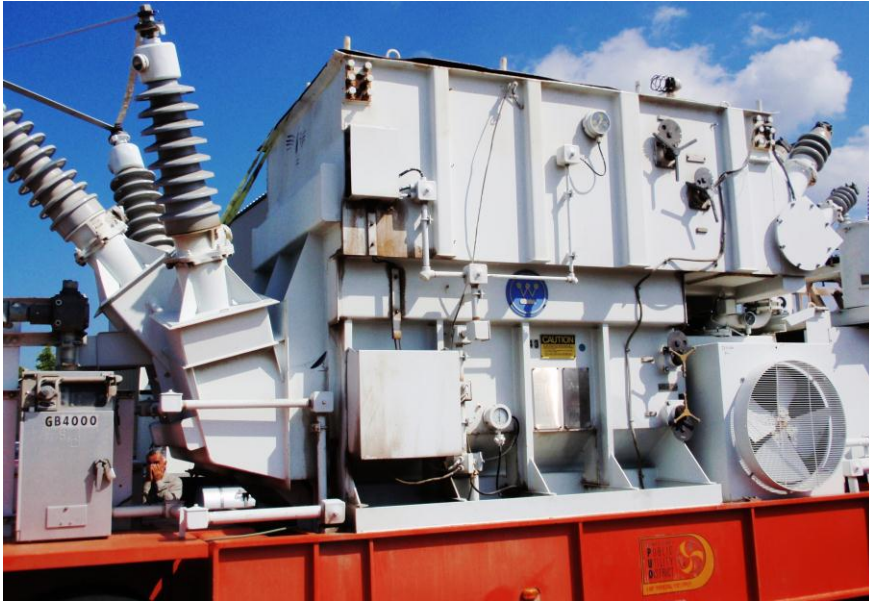
Damage to Lid from Failure Allowing Exposure to Water
