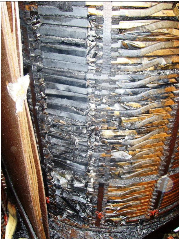
Failed Primary Aluminum Winding
