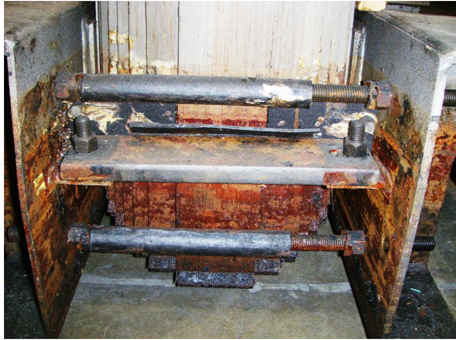
Rusted Bottom of Core Steel and Bottom Frame from Water Damage
