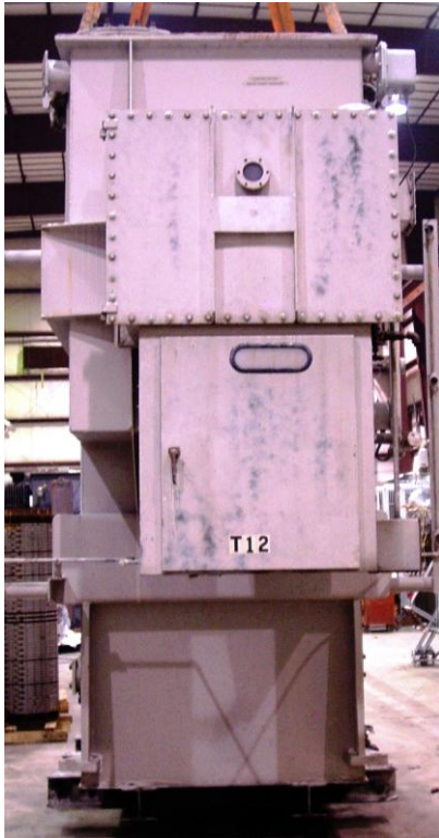
Original FPE Load Tap Changer
